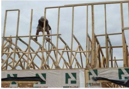
Failing to use proper fall protection is a frequently cited violation by VOSH & OSHA.
